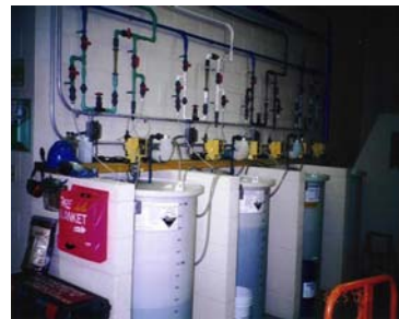
HMA Chemical Feed Room
