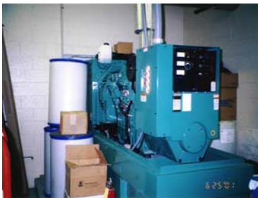
HMA Emergency Power Generator
